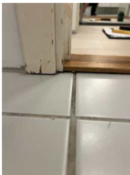
Manglende membranoppbrett under terskel
