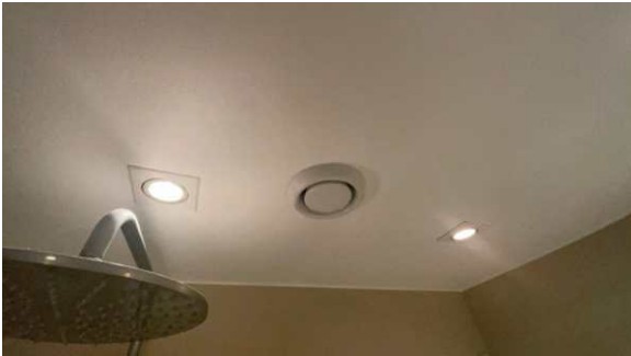
Lufteventil i himling.
