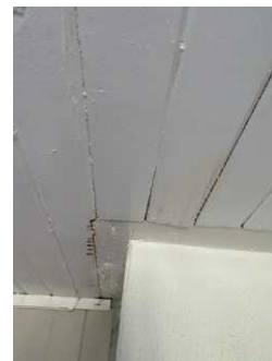
Fuktmerker i himling rundt pipe.
