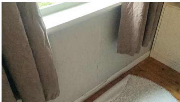
Riss i vegg under vindu
